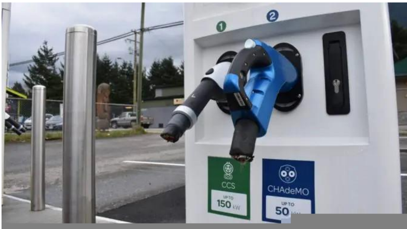
Electric vehicle charging station with severed cables.
